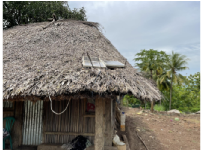
Recently installed solar panels in Cruz village, Bobonaro
